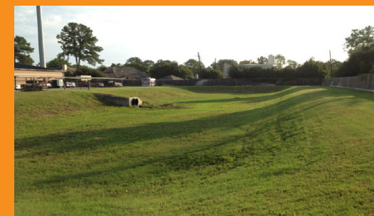
A dry detention pond: Embankments and bottom are grassed to provide erosion protection and stormwater.
