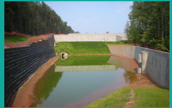
Concrete-walled dry detention pond with earthen bottom: Concrete sides provide erosion protection. The grass is well maintained with no unwanted plants. The bottom of this pond dries between storm events and indicates a well-designed and maintained detention facility.
